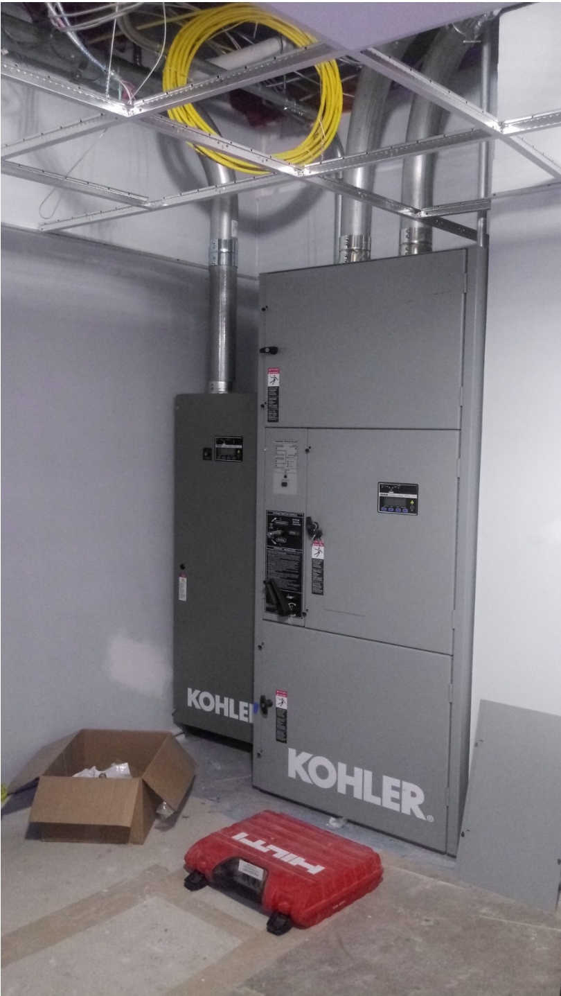
Server Room 122 – ATS & MTS Switches
